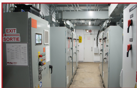
Inverters & custom instrumentation controls
