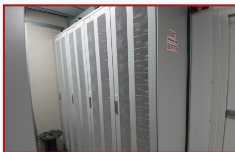
Energy storage & battery systems
